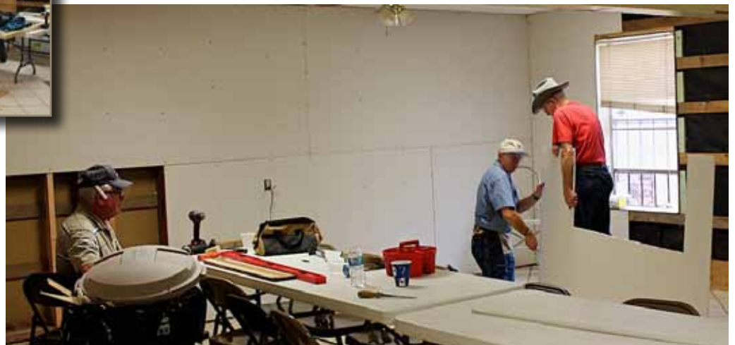
Below: Hanging the new dry wall in the Fellowship Hall. Jim Weber, Alabama, Dave Carter, Indiana, and Dave Ferris, Nebraska complete hanging the new wall.
