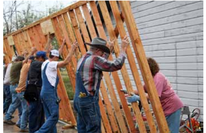
Raising the wall on the Sunday School/dormitory rooms for the Open Hands Community Ministries. Dave Ferris, Richard Binder, Ron & Deb Herrold, Cindy Dahlquist, Steve Loeschen and Bert Hendriksen are shown lifting the wall into place.
