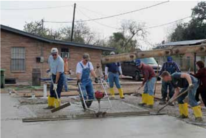
The team formed up the construction site and poured the concrete slab for the 28' X 40' Sunday School/dormitory room. Dave Carter, Richard Binder, Ernie Laird and Paul Herrold are shown screeding the pour.
