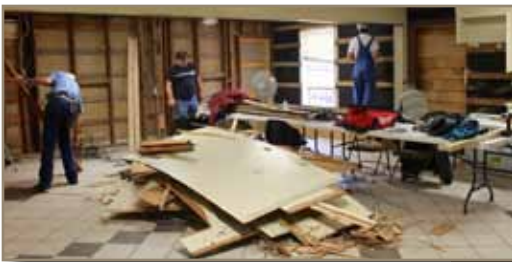
Above: Giving the walls a facelift in the Fellowship Hall at the Church in Donna, Texas. Dave Carter, Indiana; Steve Loeschen, Iowa; and Richard Binder, Nebraska tearing out the old wall board.
